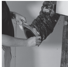
Finish by taping the vapor barrier to the collar to insure proper seal.
